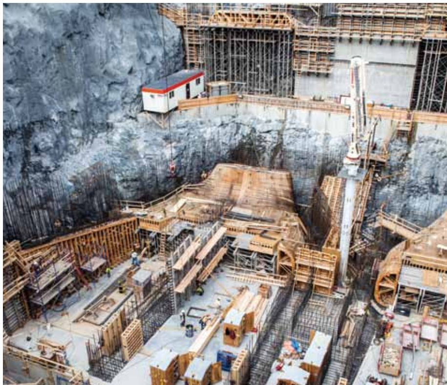
Construction has been proceeding on time and on budget at the Waneta Expansion Project near Trail.
