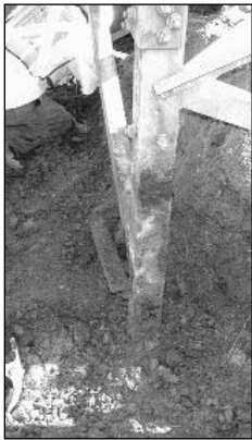
Steel tower corrosion.
