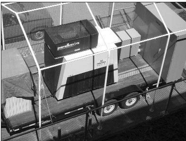
Microturbine on trailer.
