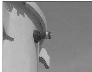
IFD™ installed transformer
