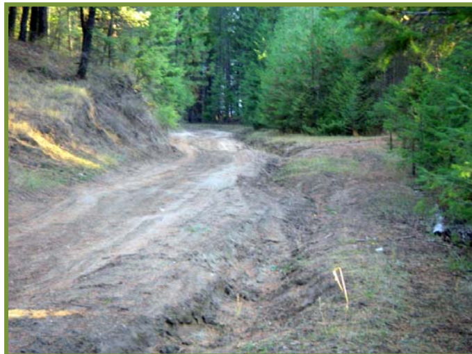
Poor vehicle access, erosion of the road bed poses a safety issue. North of Kikumon bridge northeast of Jaffray. (Source: FPB)
